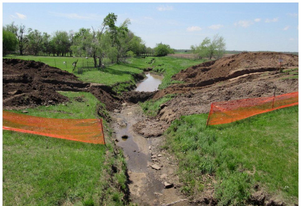
A trench has been dug across Salt Creek in Kansas, to install a pipeline. Improper management of spoils has led to silt impoundment within the stream bed, and soil stockpiles sloughing into the stream. Photo courtesy Steve Samuelson, Kansas Department of Agriculture.
