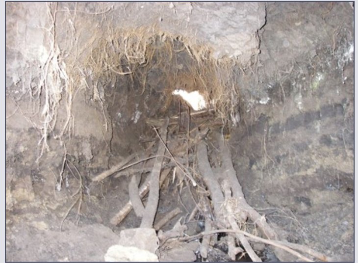
Looking inside a rodent hole that extended from upstream to downstream, entirely through a dam (Note daylight in center of photo).
