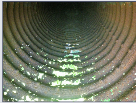
Severely corroded principal spillway pipe in Jefferson County.
