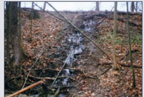
Seepage through dam damaged by tree roots. Trees should not be allowed to grow on dams. (Photo: ASDSO)
