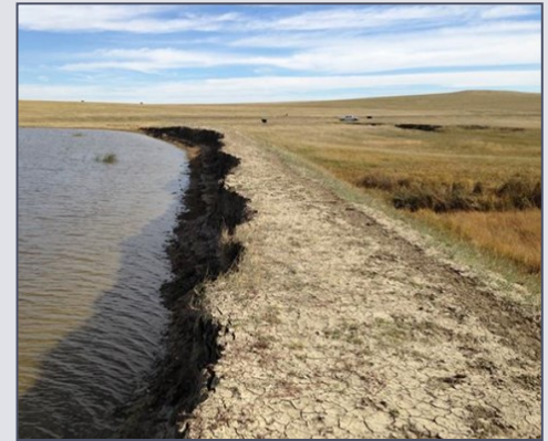
Failure to address erosion issues as they develop leads to costly repairs.
