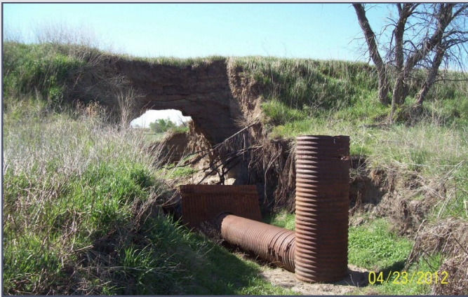
Corrosion of the corrugated metal principal spillway pipe led to this dam failure in Adams County.
