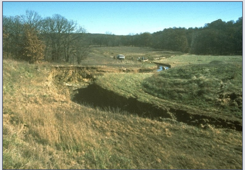
Vehicle paths in the auxiliary spillway led to failure of this dam in Kansas. Vehicle ruts and cattle trails in earthen spillways must be repaired and reseeded to prevent erosion. (Photo source: Darrel Temple)
