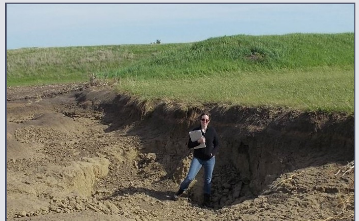
Erosion in auxiliary spillway where grass cover was removed and planted to crops.
