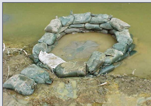
Sandbags surrounding a boil on the downstream side of a dam to pond water and create back pressure. (Photo source: USDA)
