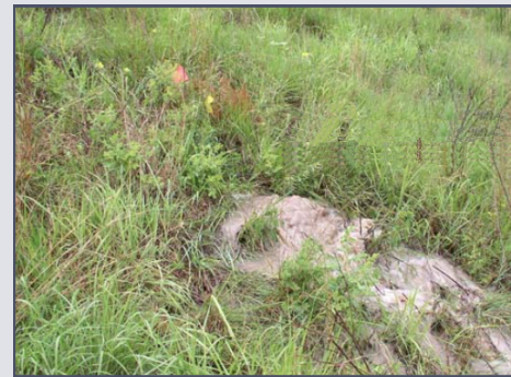
Cloudy seepage emerging from the downstream slope of dam in Frontier County, an indication that internal dam erosion was occurring. (Photo source: NRCS)
