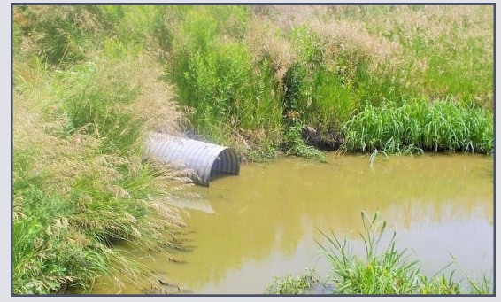
Standing water in outlet pipes accelerates corrosion of metal pipes and reduces spillway capacity.
