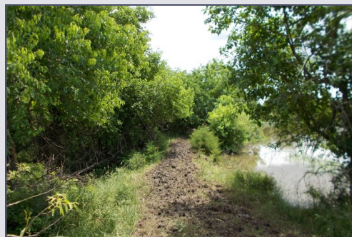
Trees make inspecting the dam difficult and provide attractive habitat for burrowing animals.
