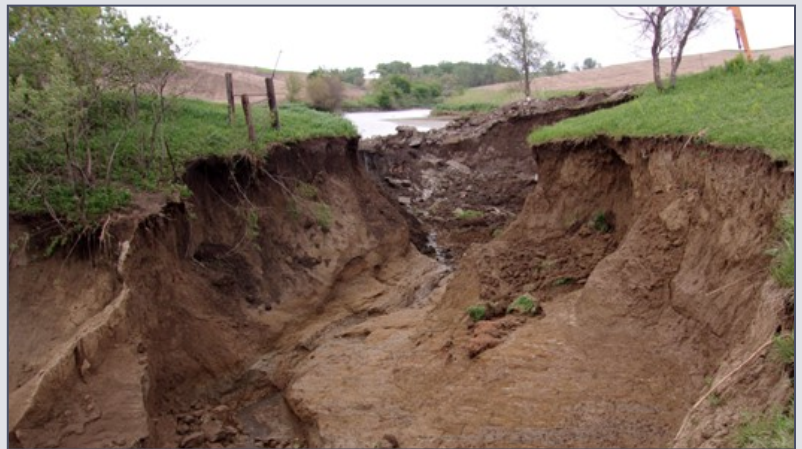
Failure of dam in Dixon County due to erosion in the vegetated earthen auxiliary spillway. A healthy, uniform grass cover is critical. One imperfection in a vegetated spillway, such as a small patch of dead grass, can be the starting point for erosion. Once erosion begins, the eroded area can quickly grow in size and breach the dam.
