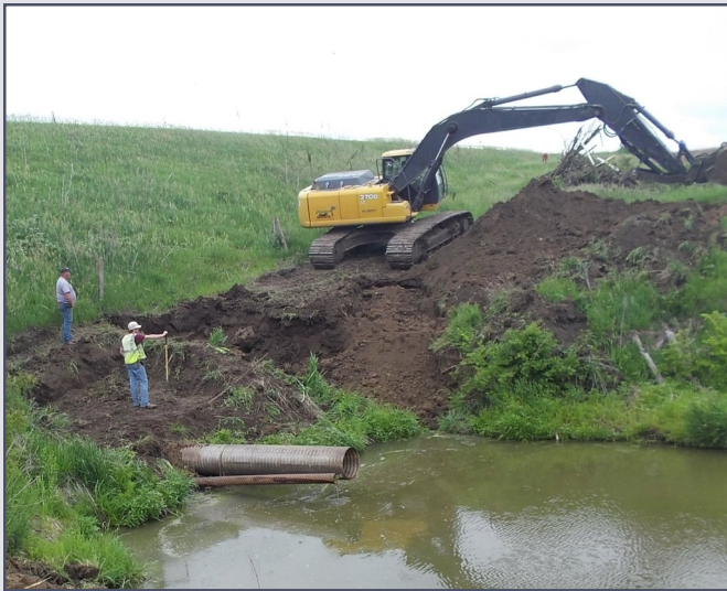
To repair damage, large rodent burrows may need to be excavated and backfilled with compacted soil.
