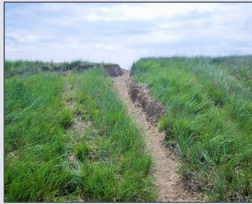
Dam embankment damaged by livestock.
