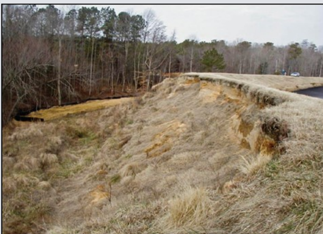
Large slide extending into the crest of a dam. Slides are typically caused by unstable steep slopes and saturated soil conditions following heavy rainfall. Slides can also be caused by rapid draining of the reservoir. (Photo Source: USDA)
