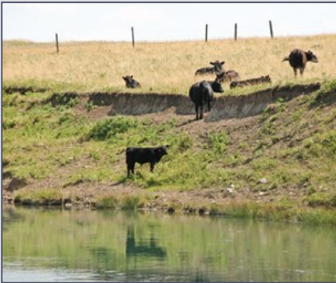
It is best to prevent livestock from grazing on dams and in spillways. (Photo source: USDA)
