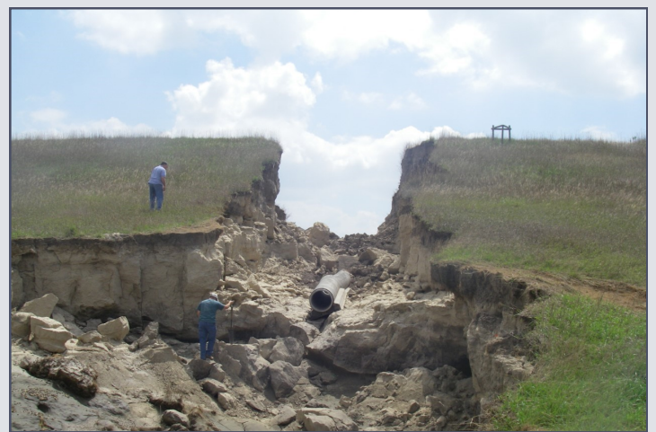
A transverse crack is believed to be the cause of this dam failure in Hitchcock County. Poorly compacted soil in the dam or in the foundation is the most common cause of transverse cracking.
