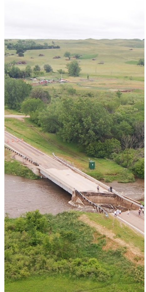
Bridge collapse caused by flooding. Photo courtesy of NEMA.
