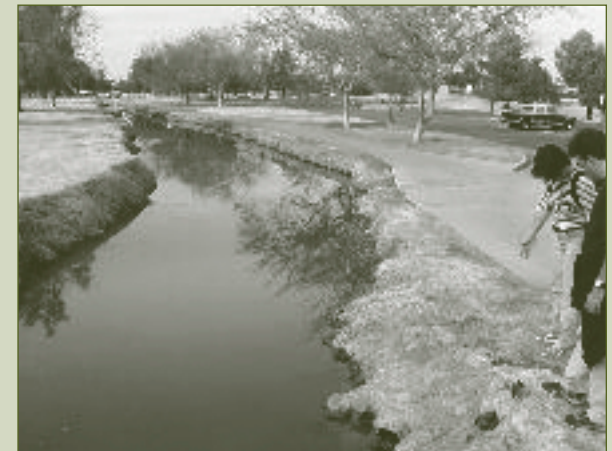
Channel wall above McKellips Street during February 2003 flood.
