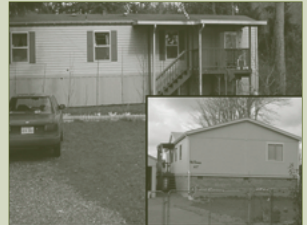
Pre-FIRM homes that are substantially improved must meet current flood zone development regulation. Each of these homes required a significant elevation change to become compliant. The elevation requirement is 2 feet above highest known historical flood elevation. In these cases, this added 3 feet to the BFE.
