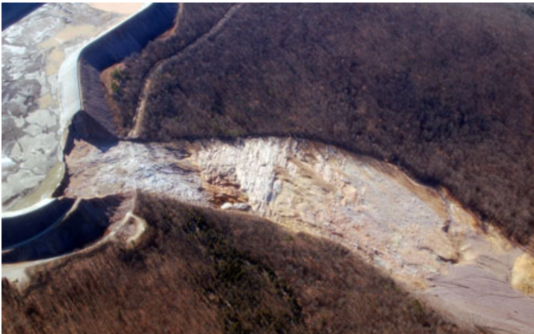
Preliminary investigation of the failure of Tom Sauk Dam near Lesterville, Missouri, on December 14, 2005 indicate that water spilled over the sides of the impoundment possibly causing erosion of the outer embankment. Source: USGS Mid-Continent Geographic Science Center.
