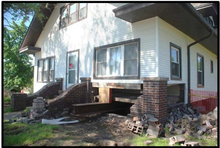
Figure 2. Basement flood damage can cause structures to collapse. Notice the steel beam supporting the upper stories on this home.
