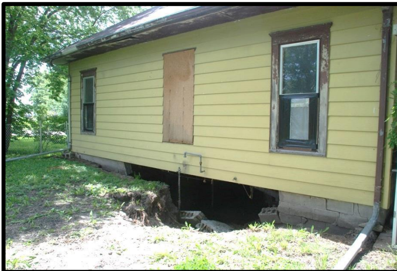
Figure 1. A home in DeWitt suffered significant basement flood damage in 2015
