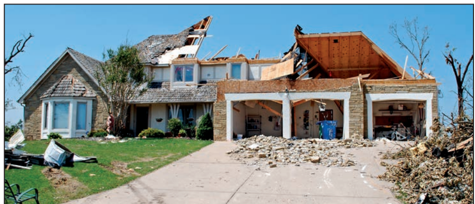
Figure 2-6: Example of a garage door failure that initiated progressive failure, including loss of the garage roof
