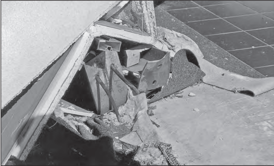
Figure B3-9. Two steel columns failed at their connection to the foundation when the anchor bolts that secured the column released from the concrete (embedment failure) while the anchor bolts that secured the column on the right experienced a ductile failure
