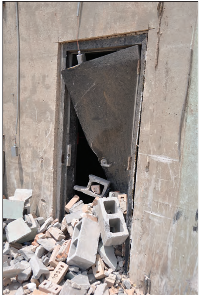
Figure B8-1. Metal door breached by wind-borne debris (this door was not designed to resist debris). (Tuscaloosa, AL, 2011 tornado)
