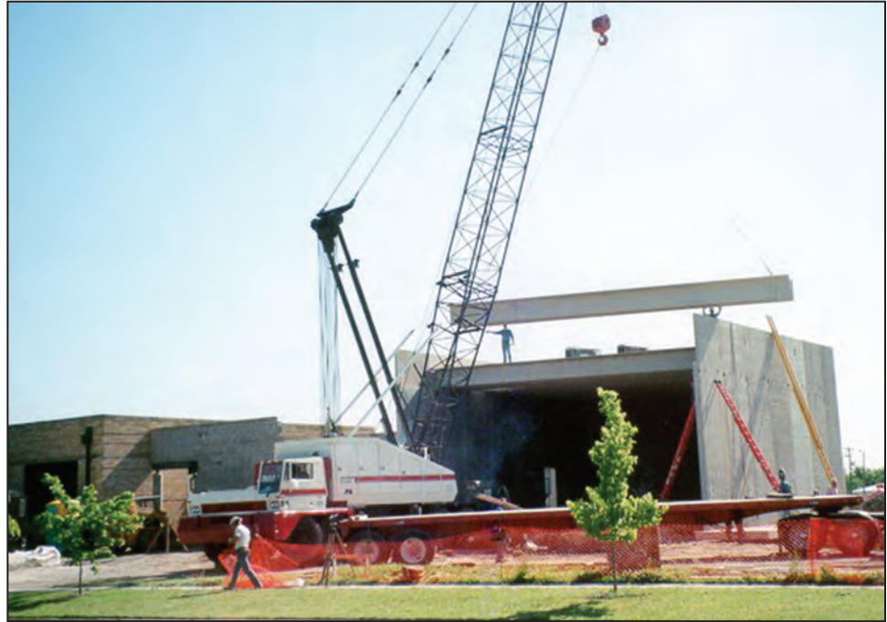
Figure B1-1. The addition to this school was designed to serve as a multi-use safe room; it is also used as a cafeteria, gym, and for large group gatherings (Wichita, KS)
