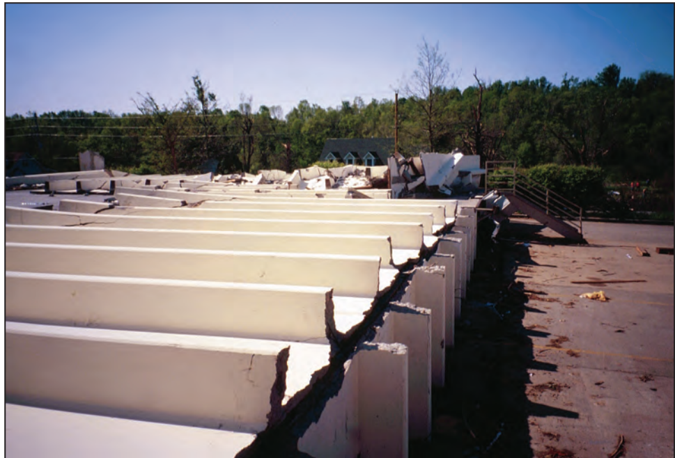
Figure B3-16. Collapse hazard: tall precast wall panels collapsed onto the floor slab (Midwest tornado, 2003)
