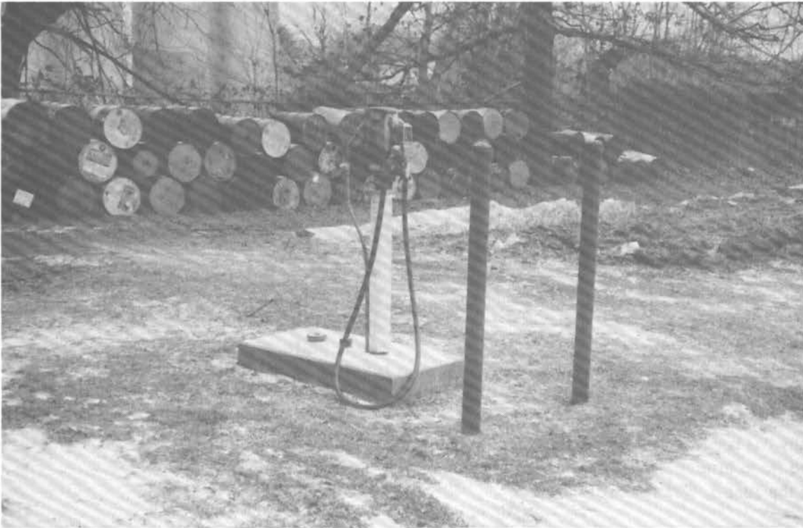
Floodproofed on-site gasoline pump to provide fuel for portable pumps and other equipment.
