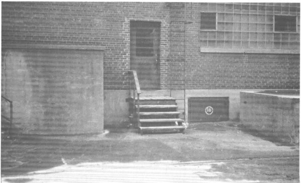
Flood shield are maintained in place over seldom-used openings.
