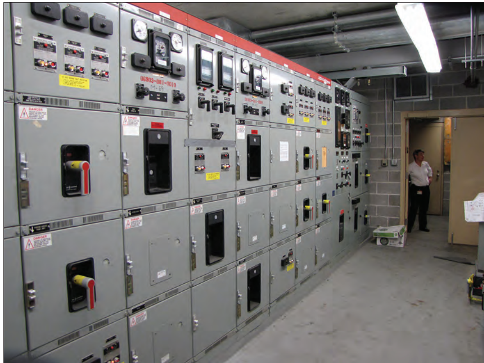
Figure 4-17. Undamaged secondary switchgear located at the University of Texas Medical Branch. The switchgear had been constructed on an upper floor that remained above flood levels. The switchgear was not damaged during Hurricane Ike (Galveston, TX, 2008).
