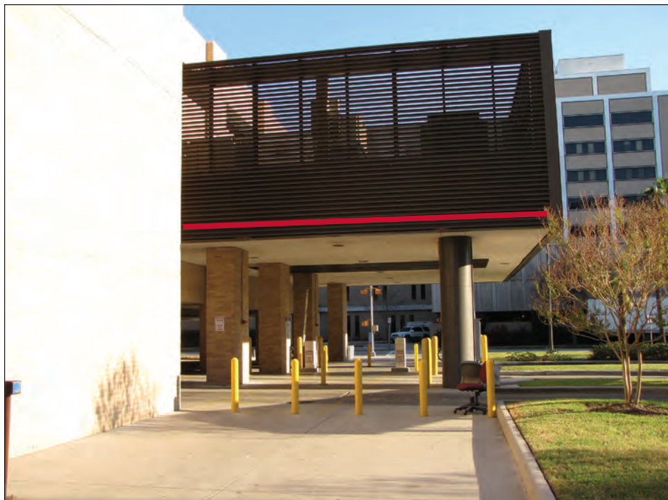
Figure 4-18. Emergency generator elevated above flood levels at the University of Texas Medical Branch, Hurricane Ike (Galveston, TX, 2008). The secondary switchgear shown in Figure 4-12 is located in the room to the left at approximately the same elevation as the emergency generator. The red line shows the location of the base of the generator.
