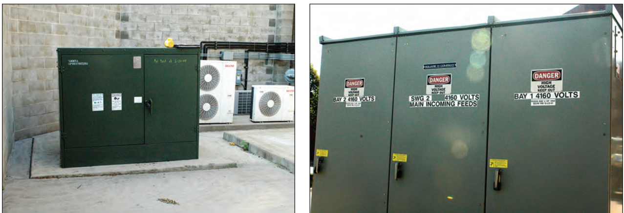
Figure 4-19. Pad-mounted transformer (left) and 15 kilovolt switchgear (right), both vulnerable to damage when inundated with floodwaters (Cedar Rapids, IA, 2008)
