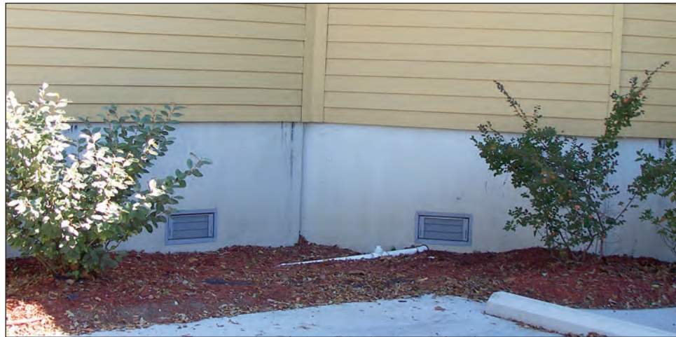
Figure 4-14. Non-residential structure retrofitted with flood openings following Hurricane Katrina (New Orleans, LA, 2008)
