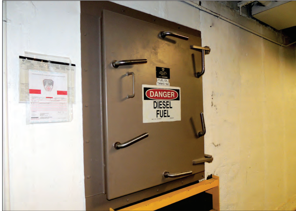
Figure 3-21. Door to a dry floodproofed generator fuel tank vault servicing multiple generators in a high-rise building
