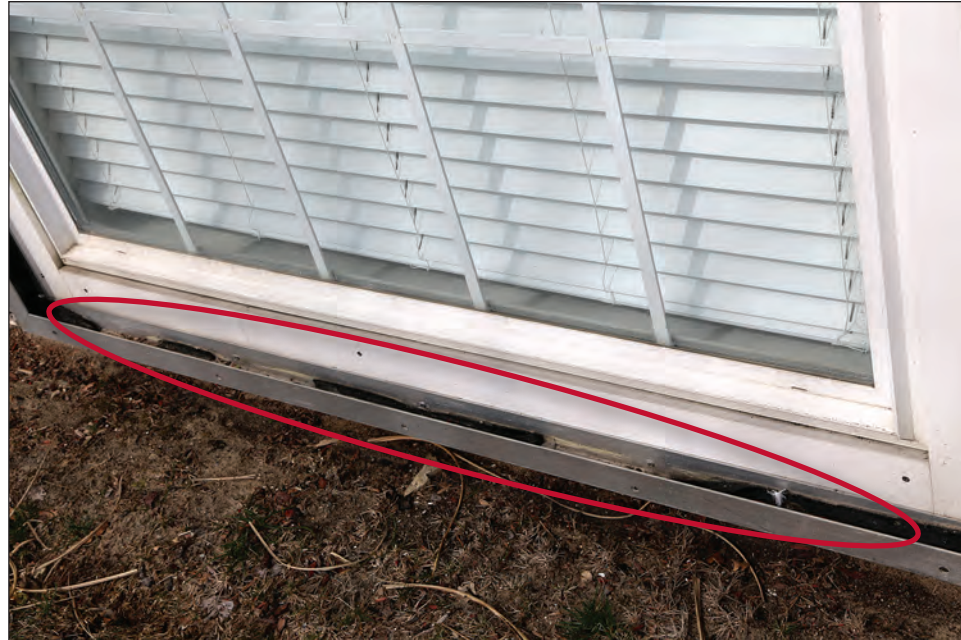
Figure 3-19. A deteriorated flood shield gasket (see red circle) that must be replaced for the shield to seal and function properly (Ocean City, NJ)
