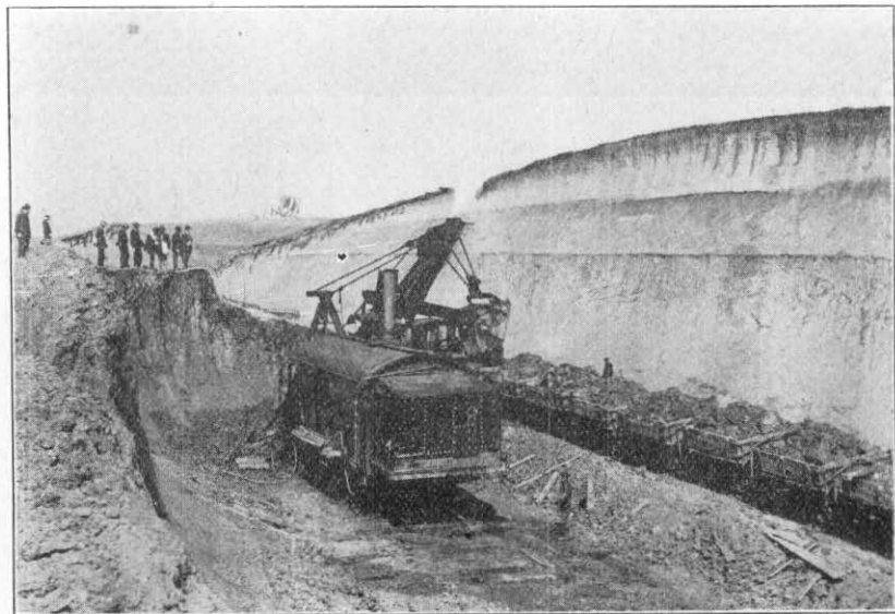
Figure 10. Railroad Cut in Drift Hills. It Is Being Widened Because of Caving. A Loess Cut Would Stand Much Better. Observe That Some of the Boulders Are Inked in.
