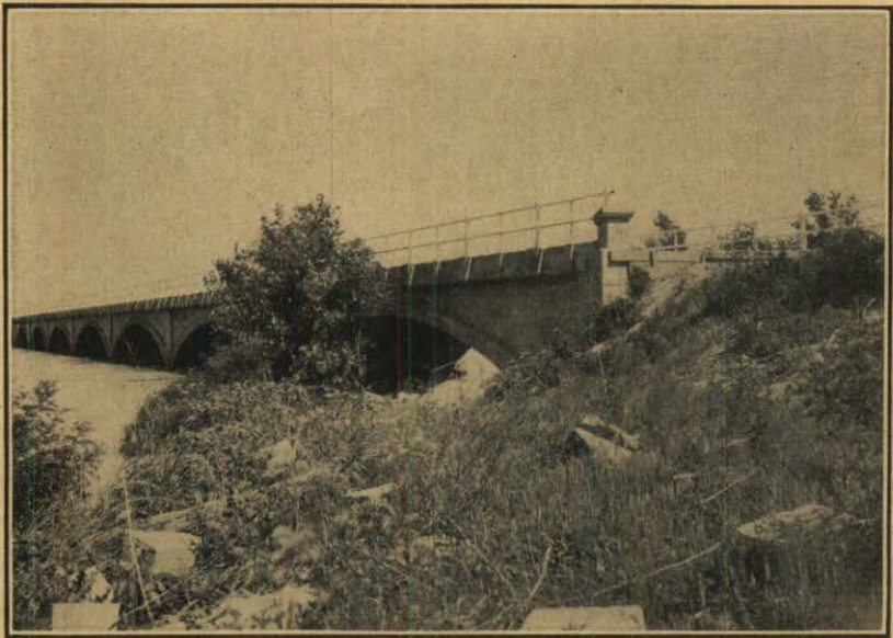
Project No. 228-C. Views of Construction—Grand Island Bridge Widening Over the Platte River.
