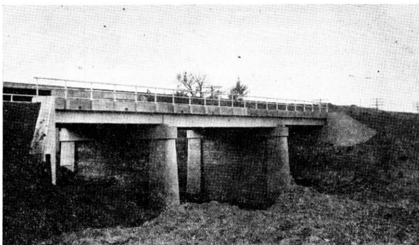
Bridge of deck steel girder type, near Greenwood on the D. L. D. Project 107-A 1.
