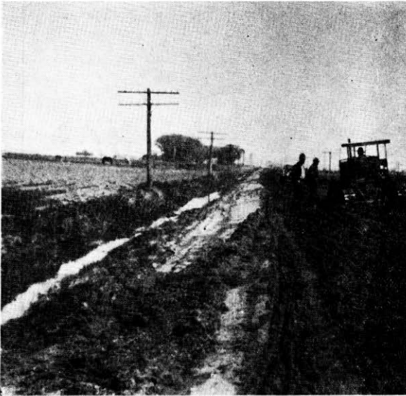
A Graveled surface was not adequate during extreme weather conditions, on this section of Highway No. 30, one mile east of North Bend, Dodge county. The gravel was replaced by concrete pavement as shown in the view below.
