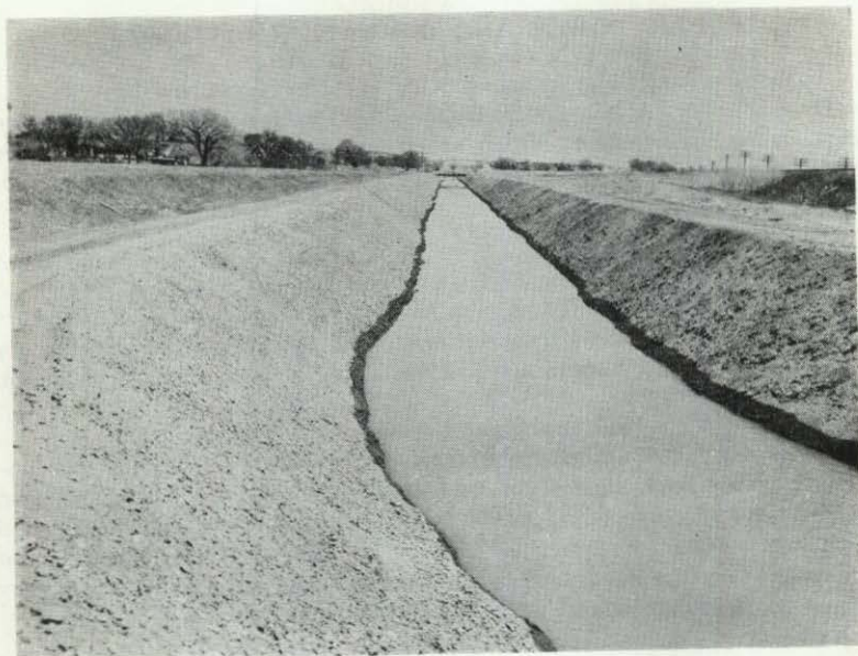
View of Cambridge Canal Near Headgate Showing First Water Diverted on April 27, 1950.
